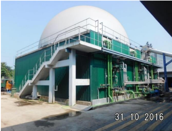
MSW dedicated biogas plant A digester module with 3 digester tanks. Total volume 1500 m 3
